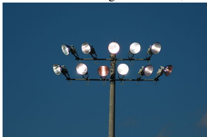
Metal halide floodlights at a baseball field
