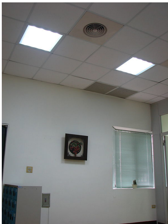
Dropped ceiling with LED lamps
