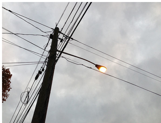
Sodium vapor street light
