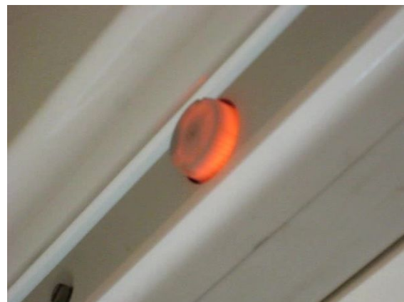
Starting a preheat lamp. The automatic starter switch flashes orange each time it attempts to start the lamp.
