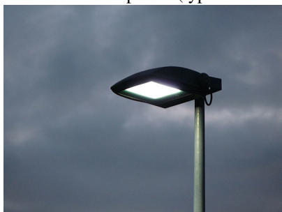
Metal halide streetlight in Tallinn, Estonia
